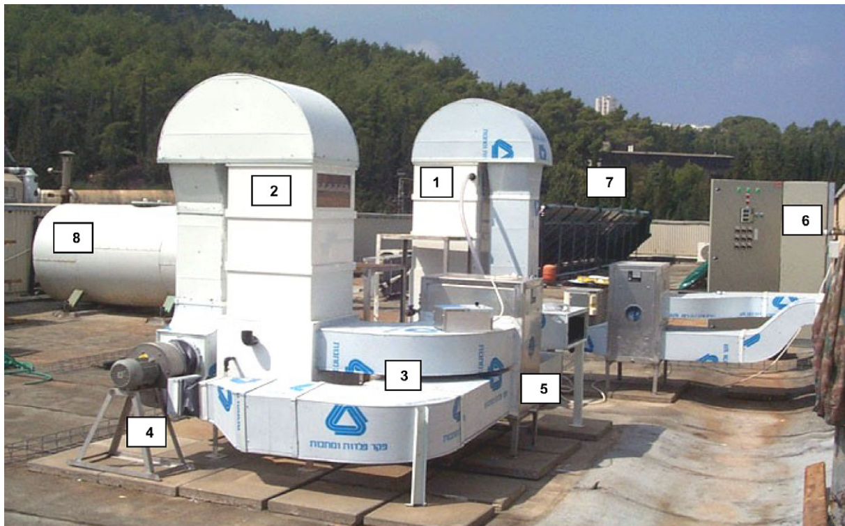
Fig. 2. Photograph of the liquid desiccant system: 1 – absorber/dehumidifier; 2 – desorber/regenerator; 3 – air ducts; 4 – fan; 5 – rotary air/air heat exchanger; 6 – control cabinet; 7 – solar collector field; 8 – hot water storage tank.
