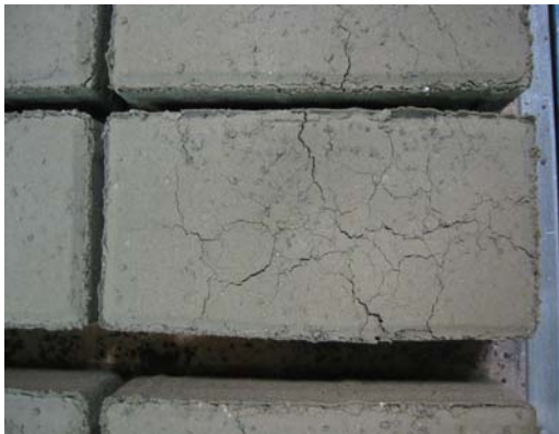
Figure 8: Cracks on paver surface
