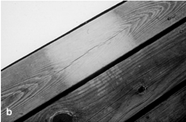
Figure 7—Removal of mildew from lumber treated with chromated copper arsenate (CCA): (a) mildew-infected board; (b) mildew removed with a bleach-water solution.
