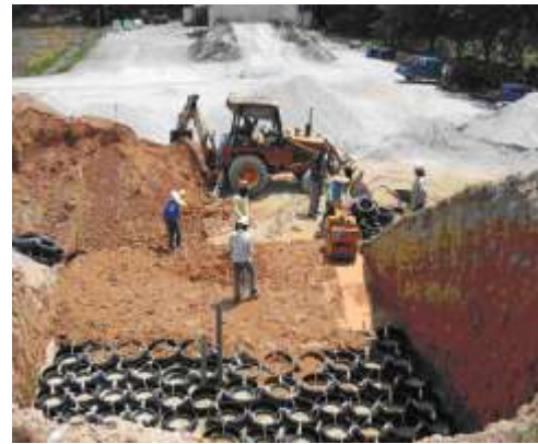
(b) Backfilling tire mat layer with in situ cohesive material and compaction
