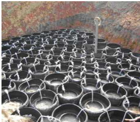
(a) Laying first tires in mat configuration, with each tire tied together with polypropylenes rope
