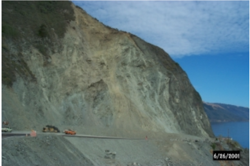
Figure 4, Debris slides above the highway at "Pitkin's Curve" may have formed due to retrogressive failure starting in a road cut.
