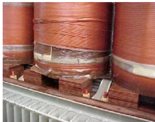
Fig.4 Primary windings of distribution transformer after a failure.
