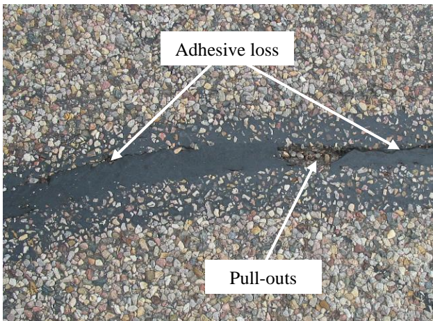
Figure 1. Sealed cracks showing two modes of failures: adhesive loss and pull-out
