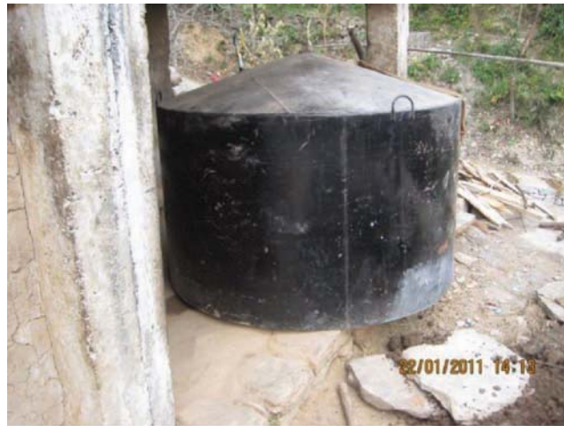
FIGURE B.7: Biogas Plant
