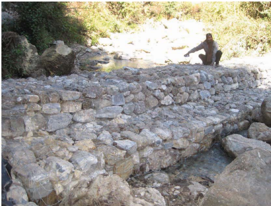
FIGURE B.2: Cratewire Check Dam
