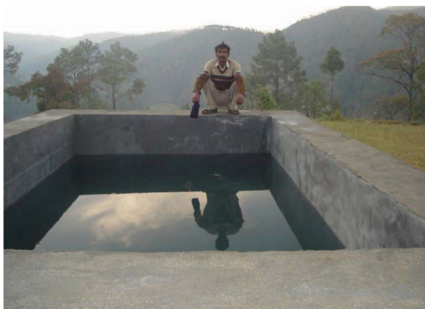
FIGURE B.6: Irrigation Tank
