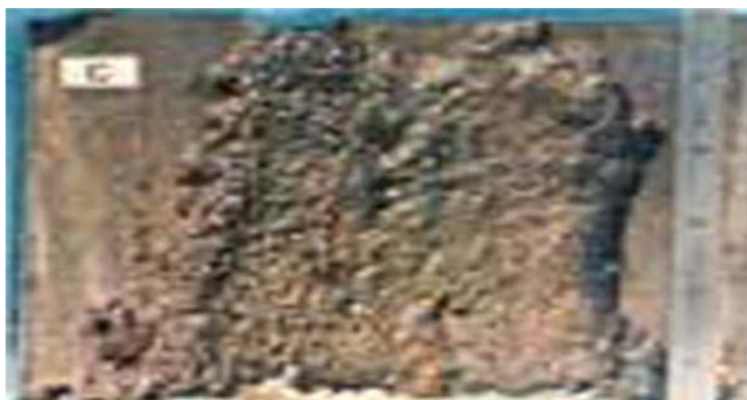
Fig.6: Internal Pipe Corrosion
