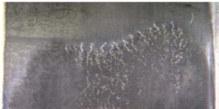
Fig.1: Crevice Corrosion in a Flange
