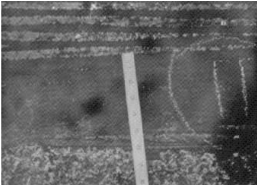
Figure 6 - Results from Runs 10 and 11. Two runs on same hull area, to eliminate gaps (as seen in top of photo from prior run). A "commercial blast", SA-2 finish was achieved here.
