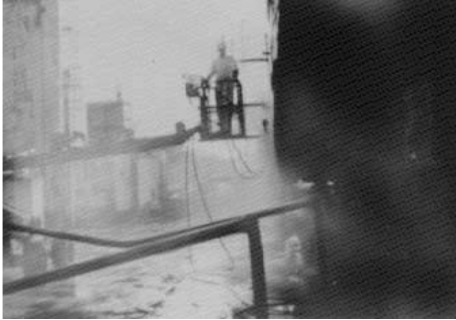
Figure 5 - "High Reach" Machine Being Driven Parallel To Ship Hull. This method of testing was used for majority of hull cleaning trials.
