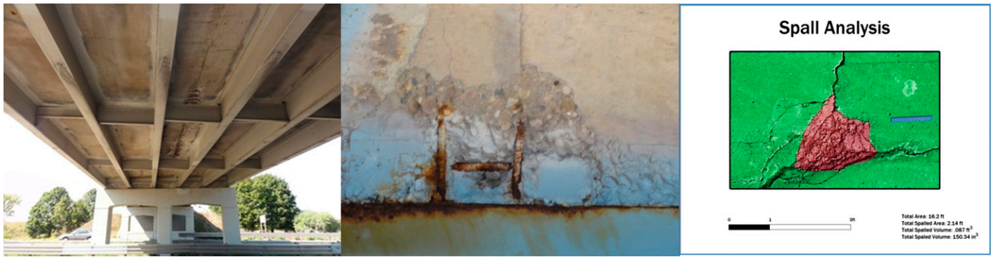
Fig. 2. Application of 3D optics for calculating the volume of spalls for inaccessible locations on the bridge deck
