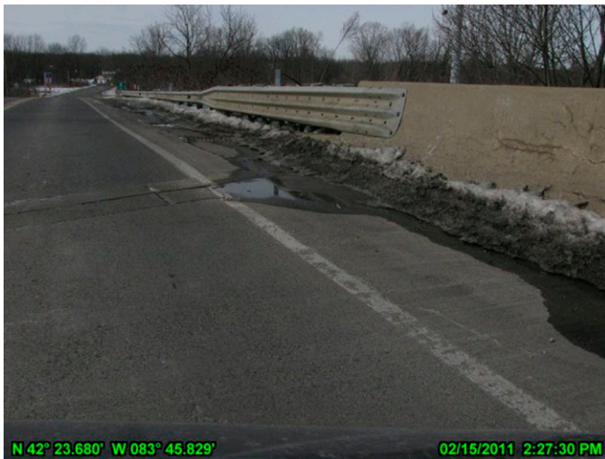
Fig. 3. Example image of part of a bridge deck taken with a bridge viewer remote camera system
