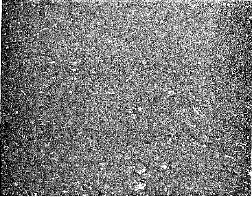
Fig. 18 - Typical texture of the bituminous base immediately after rolling. In general, the surface of this course was satisfactory, although segregation of coarse aggregate occurred at some points.
