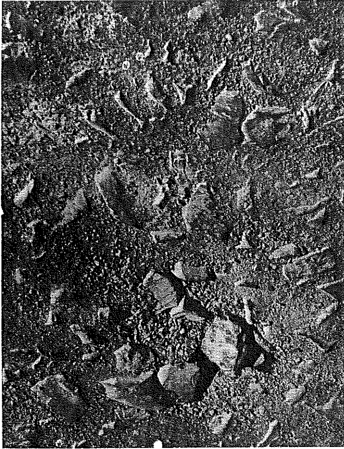
16 Fig. 16 - Localized raveling probably caused by lack of fines in the screenings. More severe cases were noted elsewhere on the road, but the condition was never severe nor worse than that of an average water-bound base constructed entirely by conventional methods.
