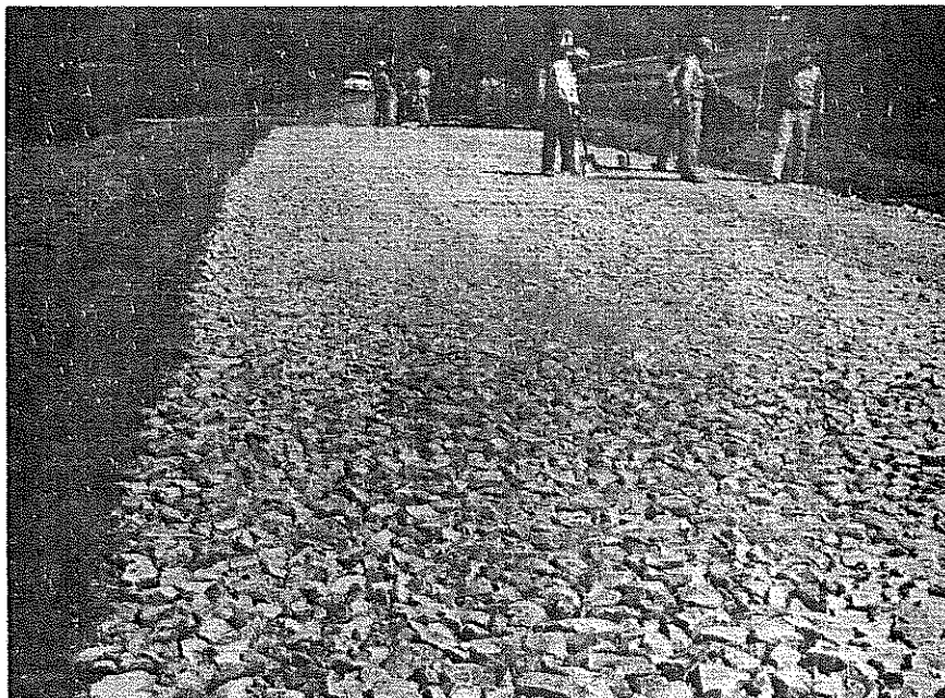
Fig. 11 - Location shown in Fig. 10 after passage of the tamper. Most of the screenings have infiltrated the coarse base stone. Note spots still covered with coarse screenings. Some difficulty was encountered where coarse screenings blocked voids and prevented complete choking of the coarse stone, particularly in the second application of screenings that followed.
