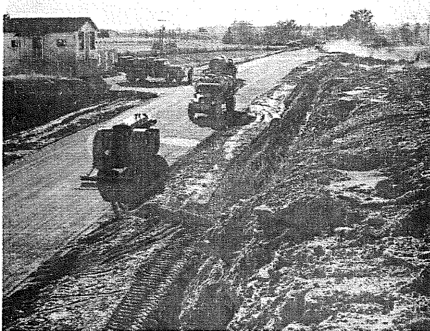
12 Fig. 14 - General view of water bonding operations. Dry brooming and rolling of the section has just been completed and sprinkling is starting. In the background the tamper is vibrating screenings on the next section.
