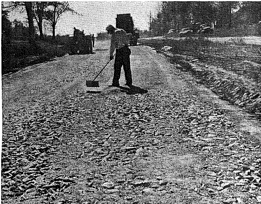
11 Fig. 13 - Location shown in Fig. 12 after passage of the vibrator over second application of screenings.
