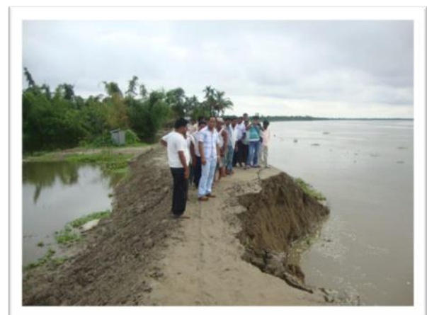
Figure 2: Breach and river erosion on the bank of river Bharamputra
