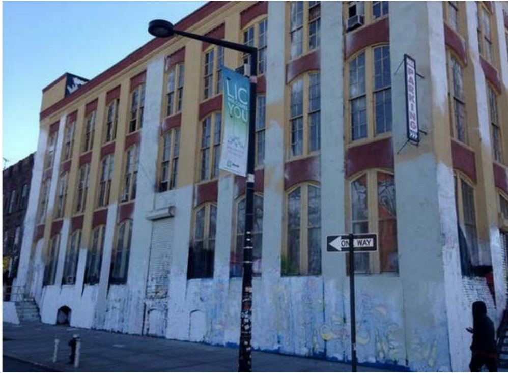
Figure 6.23: Whitewash in progress, 2013 (Breaking: 5pointz Warehouse Painted White by the Wolkoffs to, ibid. , http://queens.brownstoner.com/2013/11/breaking-5pointz-warehouse-painted-white-by-the-wolkoffs/?ic_source=ic-featured-frontpage-top .)
