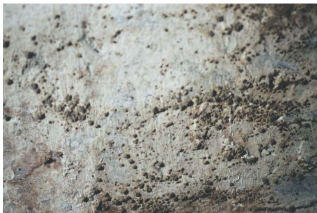
Fig. 1. The elevated fungal colonies on the lower part of the western wall as presented in side illumination. Magnification 2×.
