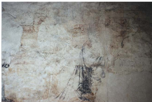
Fig. 2. The development of the discoloration is frequently coinciding with a stronger relief of the wall and could thus be misinterpreted as dust accumulations. However, as it was demonstrated by SEM, these accumulations are practically all caused by extended subaerial biofilms dominated by micromycetes.
