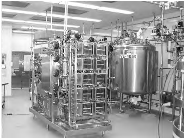
FIGURE 18.7 Virus filtration skid for processing of infliximab at the Malvern manufacturing site.
