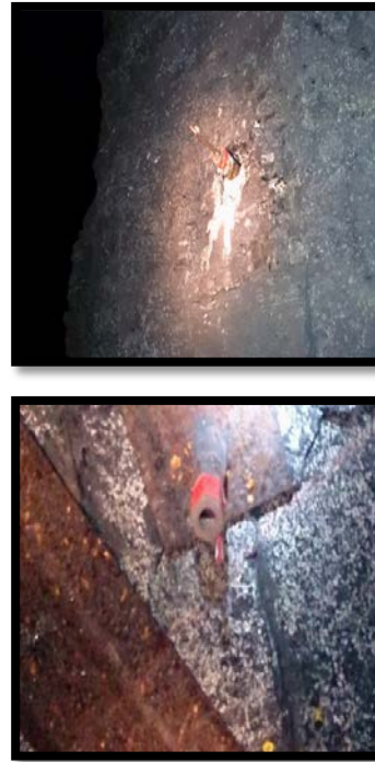
Figure 6: Rigid convergence Recorders installed underground
