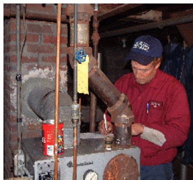
Figure 3. Yellow Tag on a Boiler
