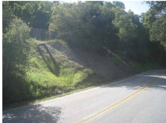
Photo 3: Western end of upper embankment below Engine Shaft. Pipe extends to shaft. Serpentinite and fill exposed in embankment
