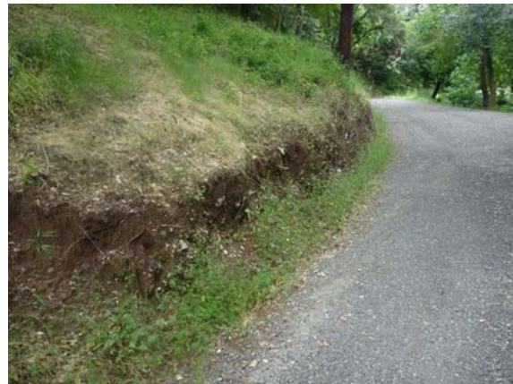
Photo 16: Road cut along Hicks Ranch Road
