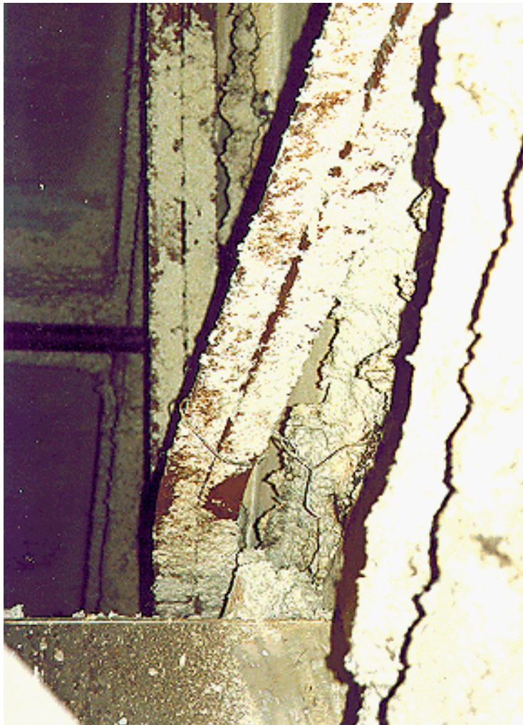
Figure 4-6. Buckled brace at the penthouse.
