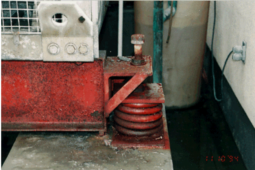
Figure 4-2. Mechanical equipment damage at the roof.
