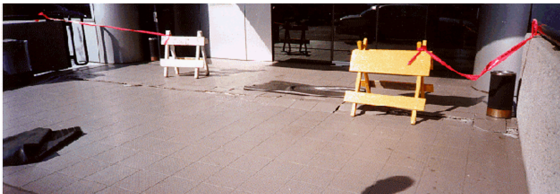
Figure 4-9. Tiles over isolation pit after the earthquake.
