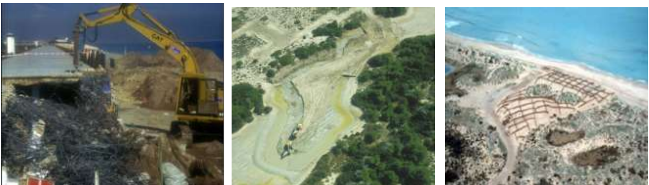
Pictures 2-4: Parque Natural de la Albufera de Valencia . Work carried out in the 1990s and 2000s in Devesa . On the left, the demolition of the existing road infrastructure ( El Saler ); in the centre, the lagoon ( malladas ) restoration; on the right, the reconstruction of the dunes ( La Malladeta ) © Ayuntamiento de Valencia, Servicio Devesa de la Albufera (2003)
