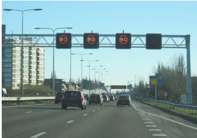
Figure 8: A variable speed limit gantry on the A13 freeway near Overschie, The Netherlands. In this particular case the maximum speed limit is 80 km/h due to environmental reasons, and the limit may drop to 70 km/h or 50 km/h in case of a downstream jam.
