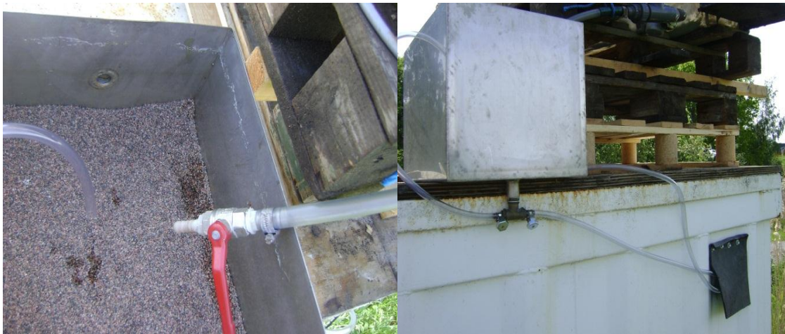
Figure 17. The sand filter and the tube from the tank are shown (left). On the end of the tube is a throttle valve. There is three tubes attached on the steel tank (right), one goes to the first column, one is for stabilizing the water level in the sand filter an and the third is for over flown water that goes to the bucket inside the container.
