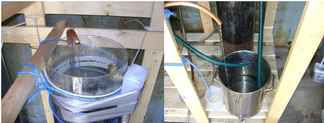
Figure 16. To the left is seen the second column with its incoming water pipe and the safety pipe. To the right is seen the tubes attached to the safety pipe that leads to a bucket where also the outgoing tube is attached in the bottom. This tube goes straight out from the container to the ditch/creek.
