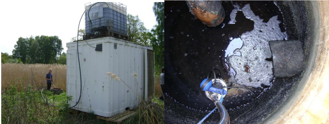
Figure 15. The pipe connected between the pump and the tank as well as the tube from the tank to the columns through an opening in the container (left). A close look in the sludge well and the pump can be seen (right).
