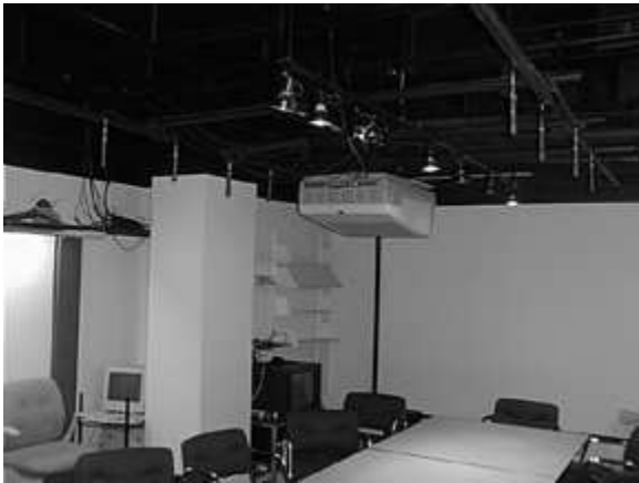
Figure 1: There are eight microphones hanging from the lighting grid in the conference room.
