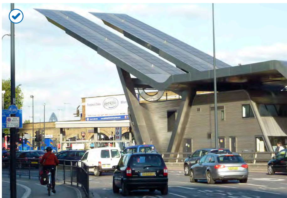
Solar panels installed on the roof canopy power the lighting for this bus exchange. Vauxhall, London, UK.
