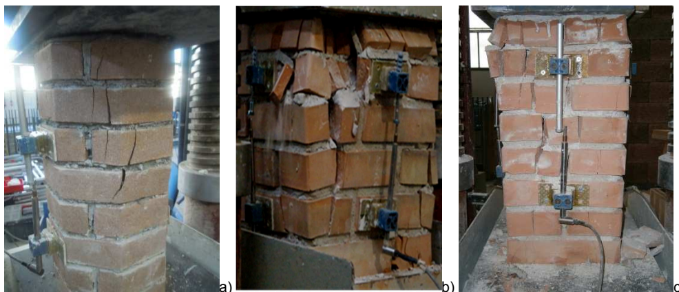
Fig. 5 Failure modes of unconfined specimens: a) Octagonal column; b) Square column; c) Rectangular column
