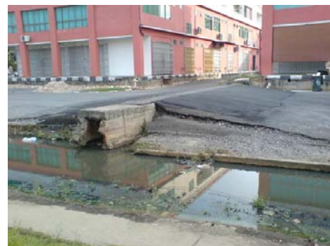
Fig. 2 Ground settlement caused poor drainage and road system in a commercial lot, Sibü.
