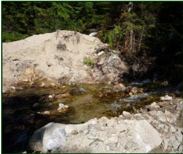
Figure 4. Unsound practice: This figure shows a section of road that was deactivated, including the removal of stream crossing structures. Investigators observed that soil was placed immediately adjacent to the channel. Some of the soil had been eroded into the stream.
