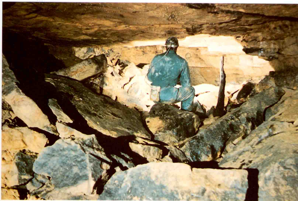
Plate 3 Roof collapse in Basal Permian Sand mine: Redhill, Castleford [441 249] (photograph by J. Hodgkins)
