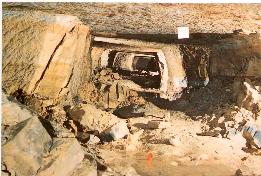
Plate 4 Deterioration of Basal Permian Sand pillars by spalling: Redhill, Castleford [441 249] (photograph by J. Hodgkins)
