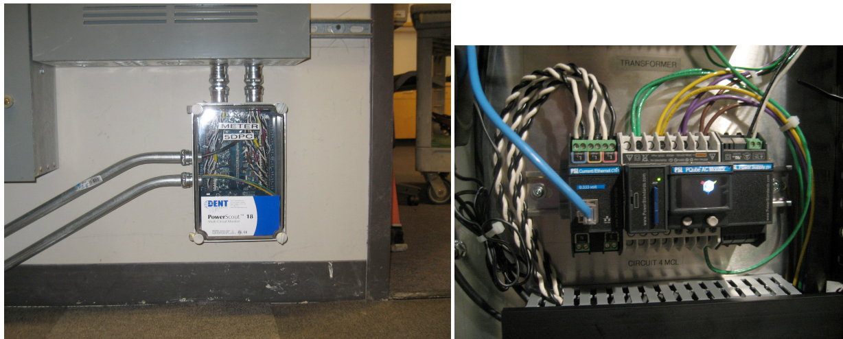
Figure 11: Left: Typical Dent installation. Right: One of two PSL PQube power meters.
