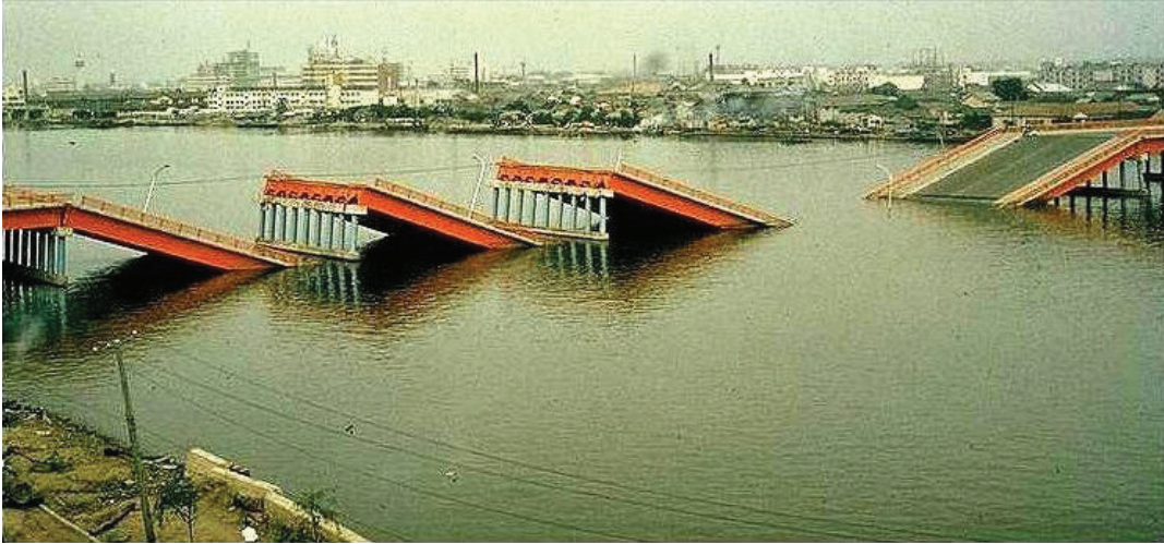
Figure 4. Collapse of the Showa Bridge after 1964 Niigata earthquake.(Source: NISEE)
