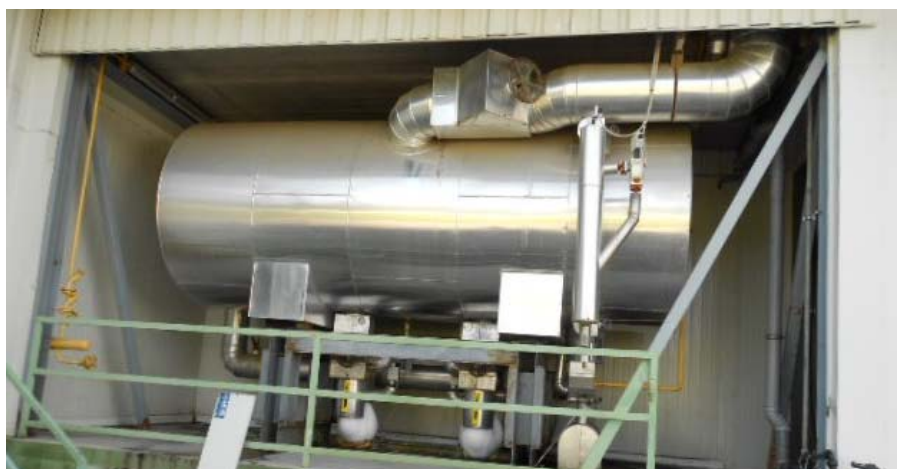
Fig. 1 Ammonia tank (directly next to the neighboring dwelling-house)
