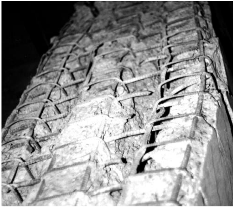
Figure 1. Pictures of fragment damage of a reinforced concrete slab caused by a cased munition.
