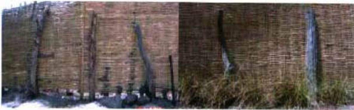
Enclosure with no vetiver has significant evidence of termite infestation - mud tunneling.
