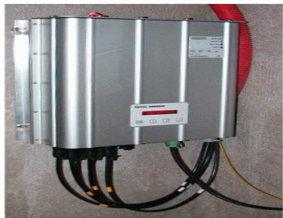
Figure-7 Electronics Inverter
