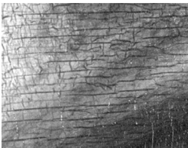
Figure 22: Horizontal cracks (veil).
