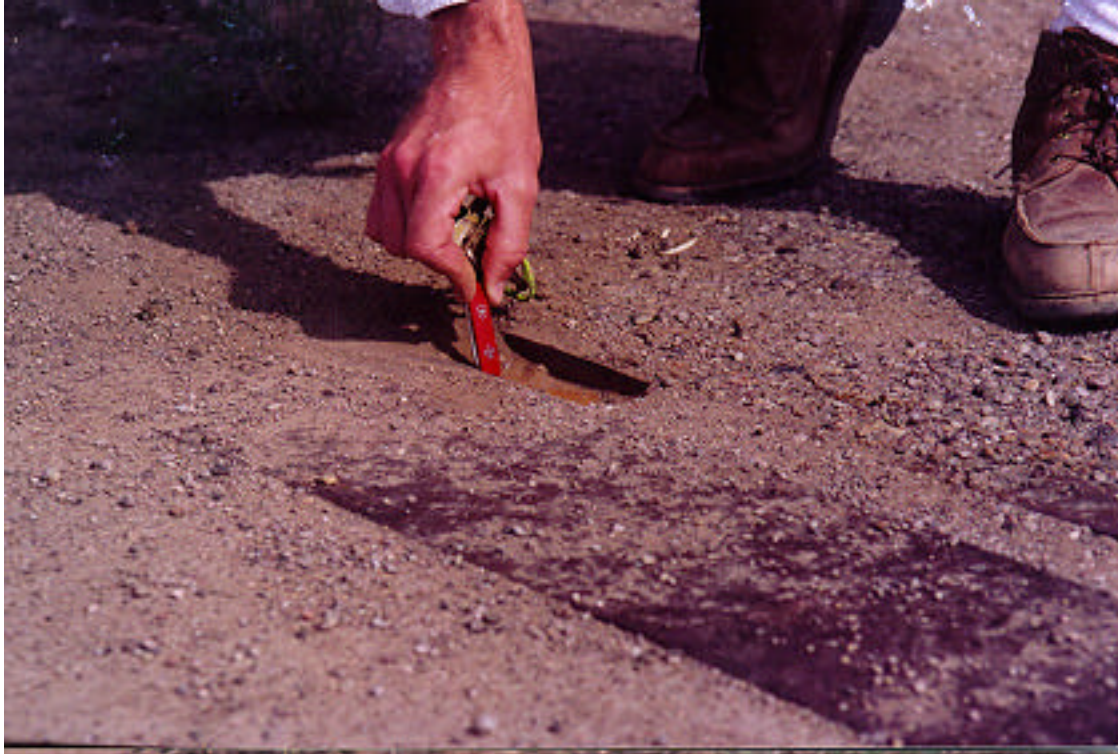
Figure 5 Debris in expansion joint.
